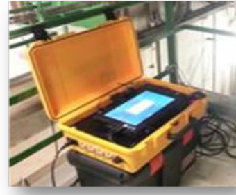
Centralized Yellow Smart Box
